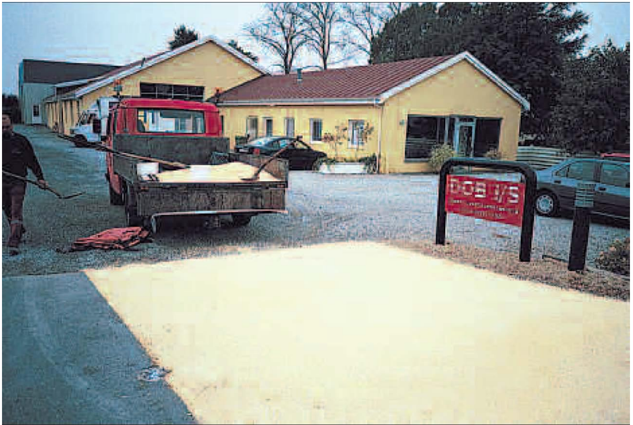
A coloured asphalt top layer with Collux® orange. The picture shows a ramp, passed by lorries every day.
